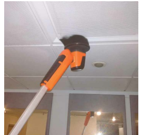
Ceilings & Ventilation Grilles
